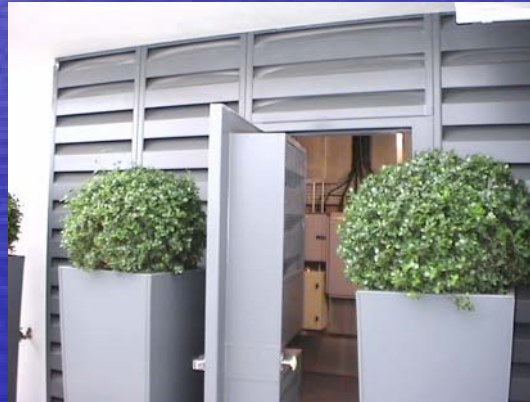
Acoustic Louvred Screen and door to condenser plant – Church St
