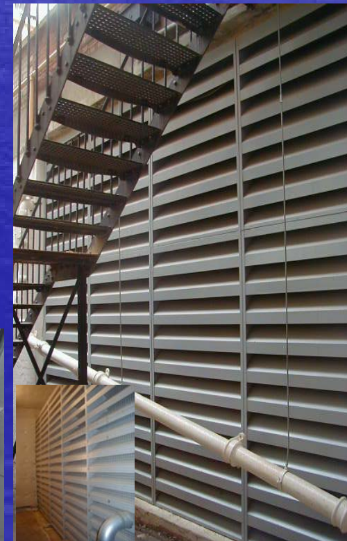
Plantroom acoustic louvre and internal view
