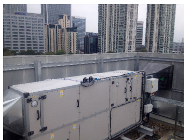
Internal View of plant screen with standard AP75 acoustic panels and supporting steelwork
