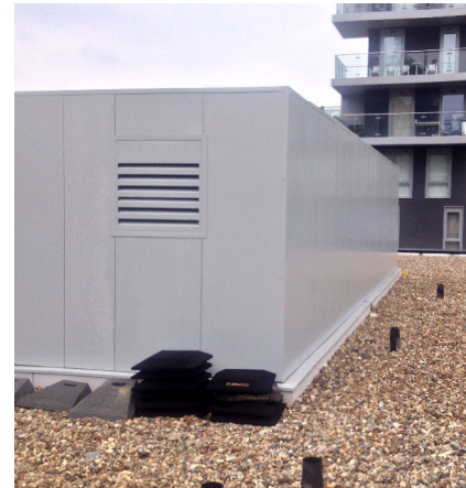
External View of plant screen with standard AP75 acoustic panels
